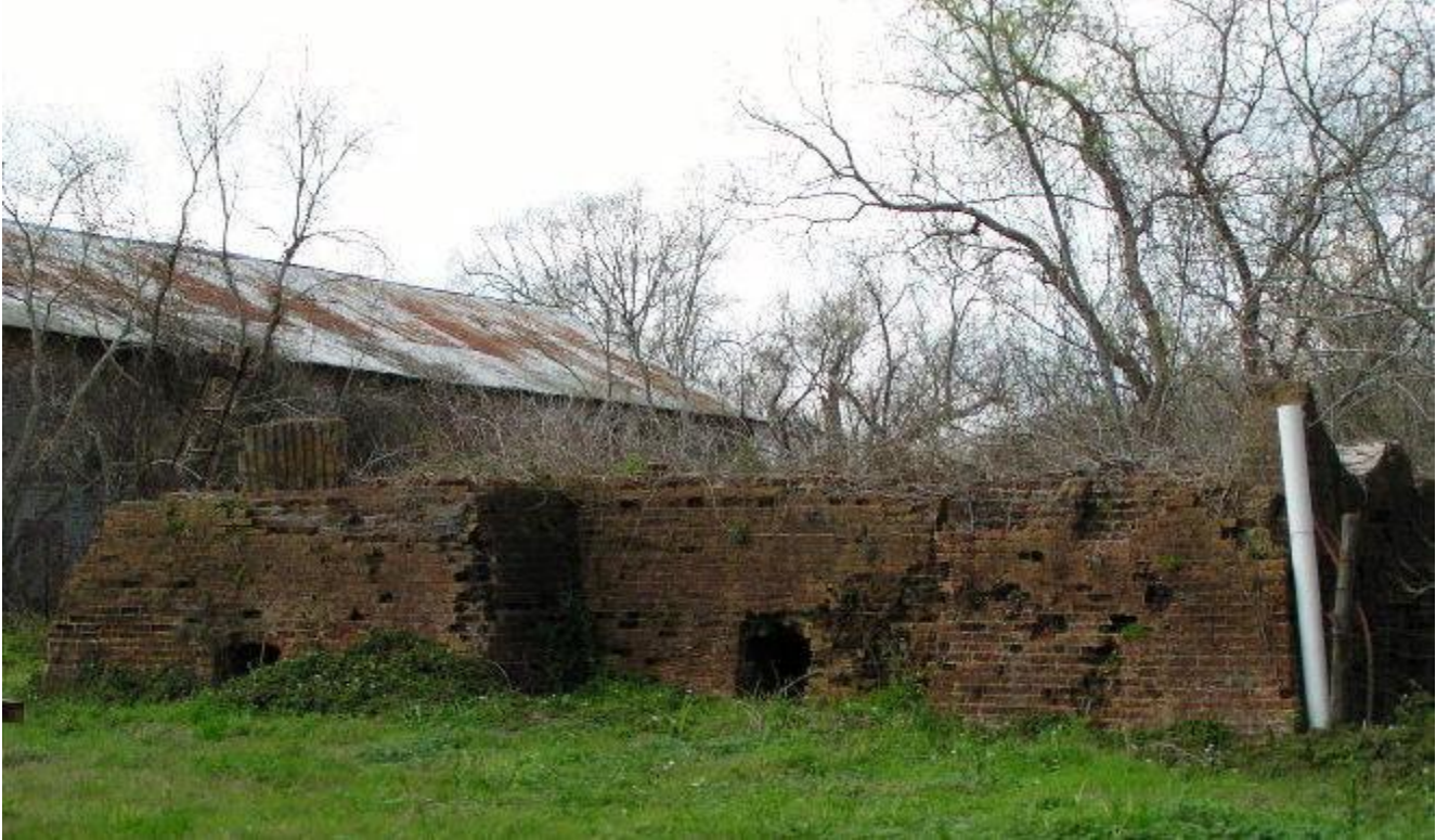
The above view is the east side of the 1840's Hartwell Iron Works Steam Engine foundation.
